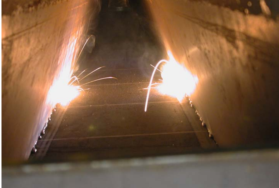
Figure 2.6 View of Weld Melt-through Inside of Rib
