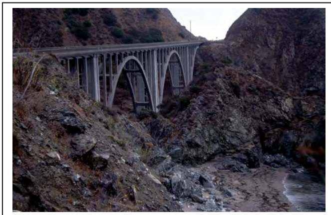
Figure 19: The concrete arch bridges, like this one over Rocky Creek, provide some of the most dramatic and memorable images of the Big Sur Coast
