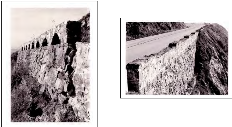
Figure 21: These retaining walls built as part of the original highway construction illustrate the arched window (left) and crenellated parapet wall designs. (Photos: Bob Pavlik)
