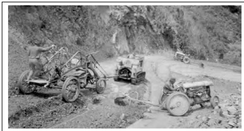
Figure 2: Removing landslide debris from the highway began even before the original construction was completed.
