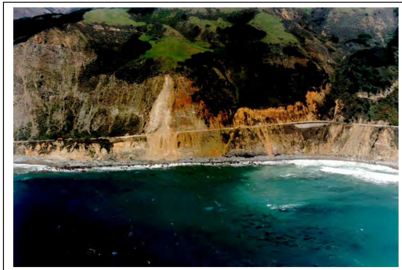
Figure 23: A landslide above the road south of Big Creek temporarily closes the highway in 2000.
