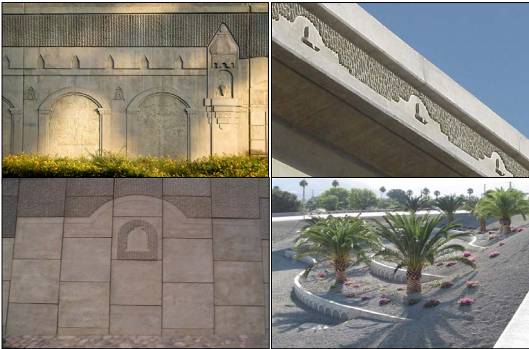
The aesthetic treatment concept used for the retaining wall (top left) was repeated in the bridge barriers, MSE walls, and low landscape retaining walls to help unify the overall highway corridor aesthetics in the City of Riverside.
