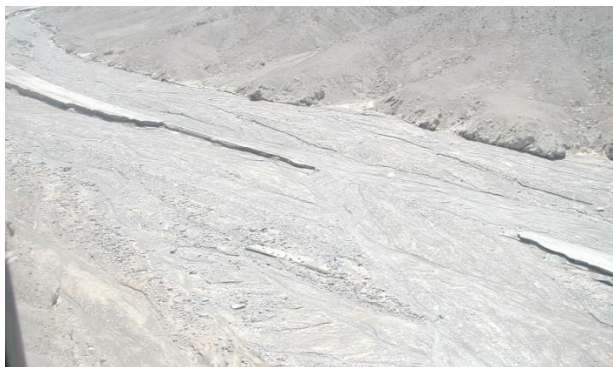
Road washout due to longitudinal location in desert wash channel
