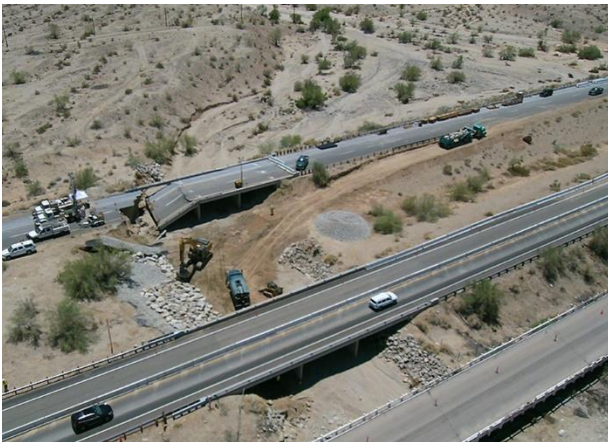
Bridge Abutment Failure at Tex Wash on I-10 after a Flood Larger Than the Design Flood
