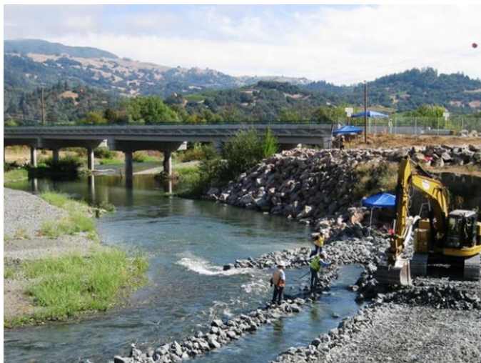
Longitudinal Peaked Stone Toe Protection (LPSTP) with Rock Vanes for Chinook Salmon Habitat Enhancement, Route 128, Russian River Bridge in Geyserville
