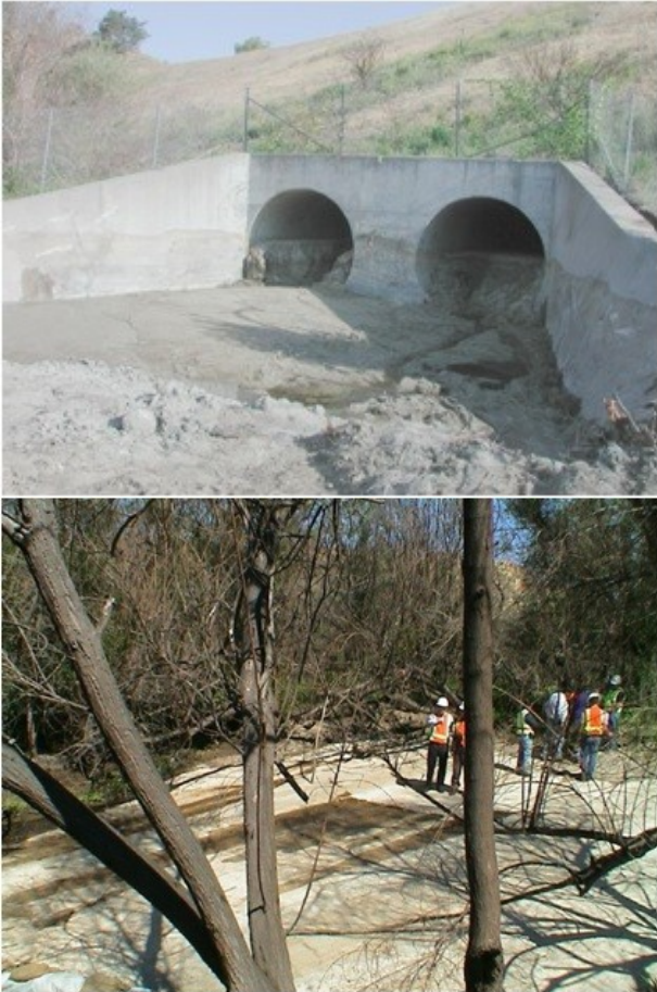
Alamos Canyon, Ventura County, post-fire debris and plugged culvert barrels (Highway 118)
